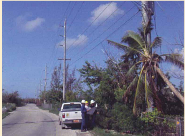
Concrete poles after Hurricane Ivan
